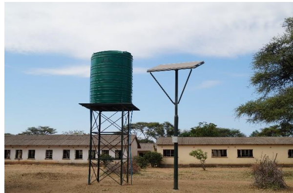
Water tank and solar pump
