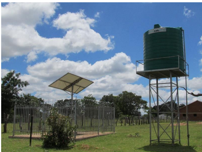
The New Solar-Powered Borehole
