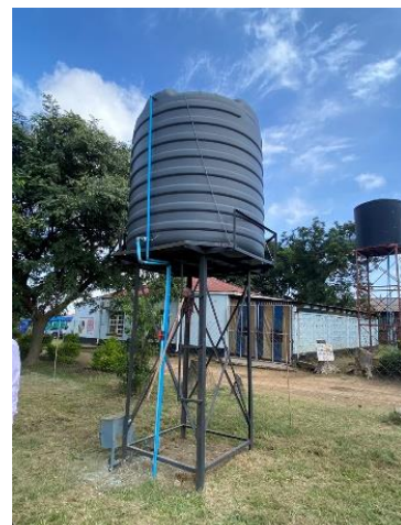
Water tank connected to the new borehole
