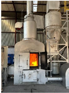
Medical Waste Incinerator
